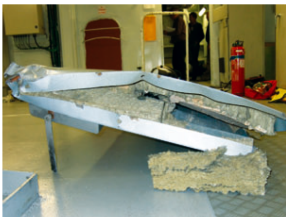
Mangled steel door from the aft main switchboard room Source: MAIB SAFETY BULLETIN 4/2010, www.maib.gov.uk
