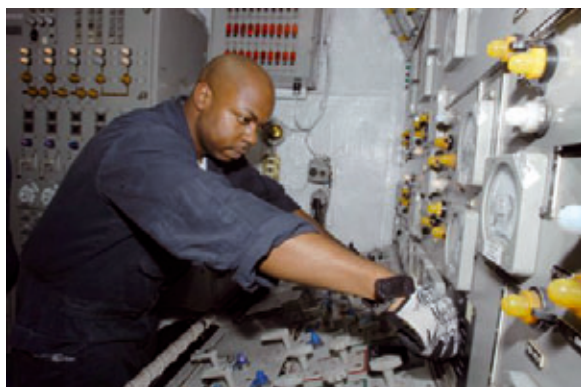
Partial view switchboard
